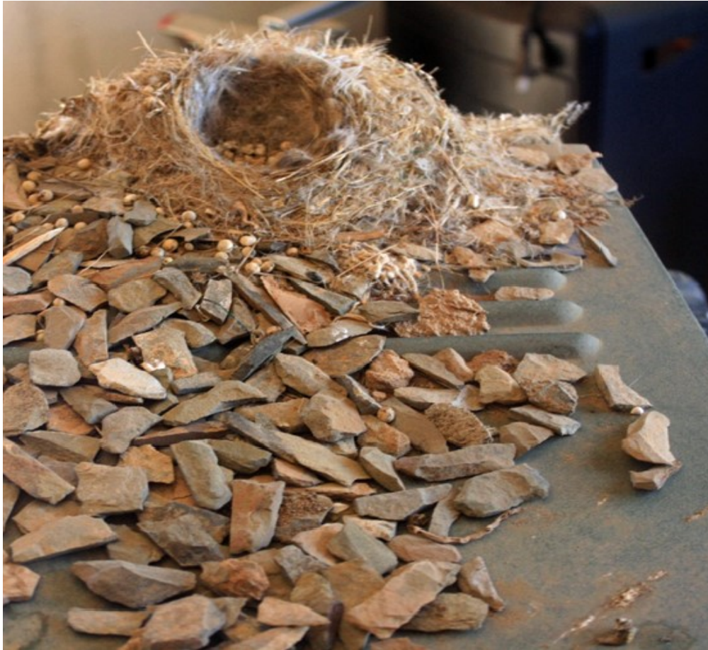
Figure 1: Nest under shelf in generator room (indoors).
