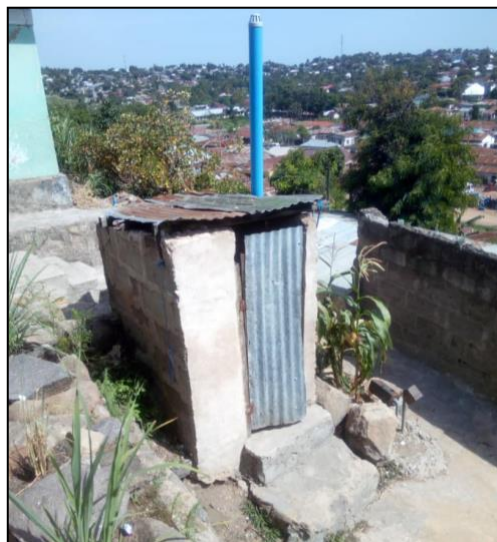
Figure 3. Toilet to be connected to a sewer
