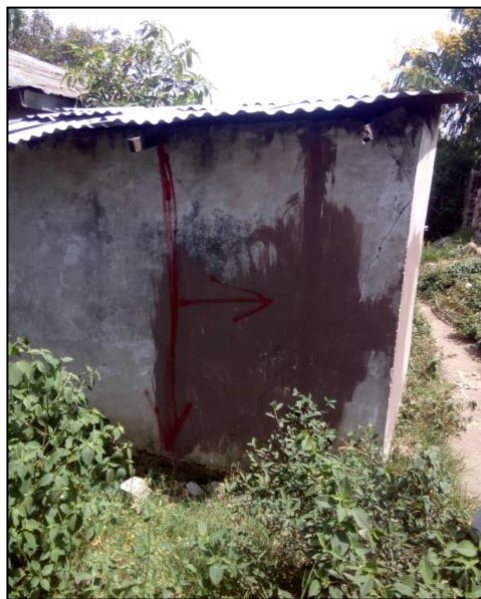
Figure 2. Land reserved for a 4m road with Part of Building to be Demolished
