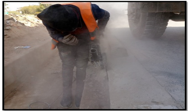
Figure 4: Picture showing dust exposure during dry concrete grinding
