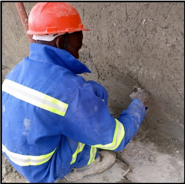
Figure 14: Picture showing a worker without gloves and a dust mask
